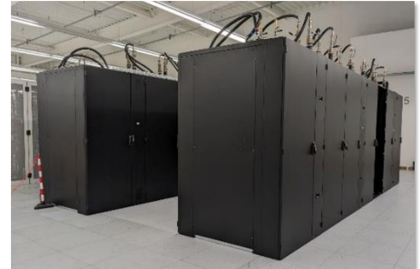
Hardware overview on IT Center Help
